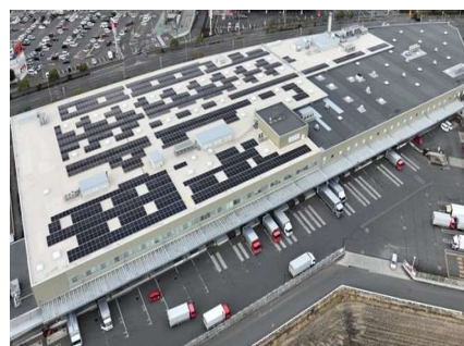
Solar power facility (Shin-Sendai Post Office)
