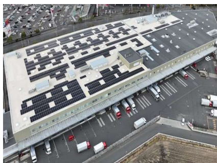
Solar power facility (Shin-Sendai Post Office)
