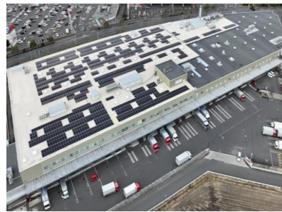
Solar power facility (Shin-Sendai Post Office)
