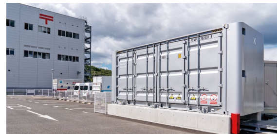
Okayama Post Office (Okayama Prefecture) has introduced a power optimization service utilizing large-scale battery storage systems
