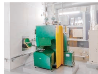
Boiler for thermal use of wood chips
