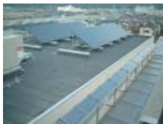
Solar energy generation panel on roof of Odawara-Higashi Post Office
